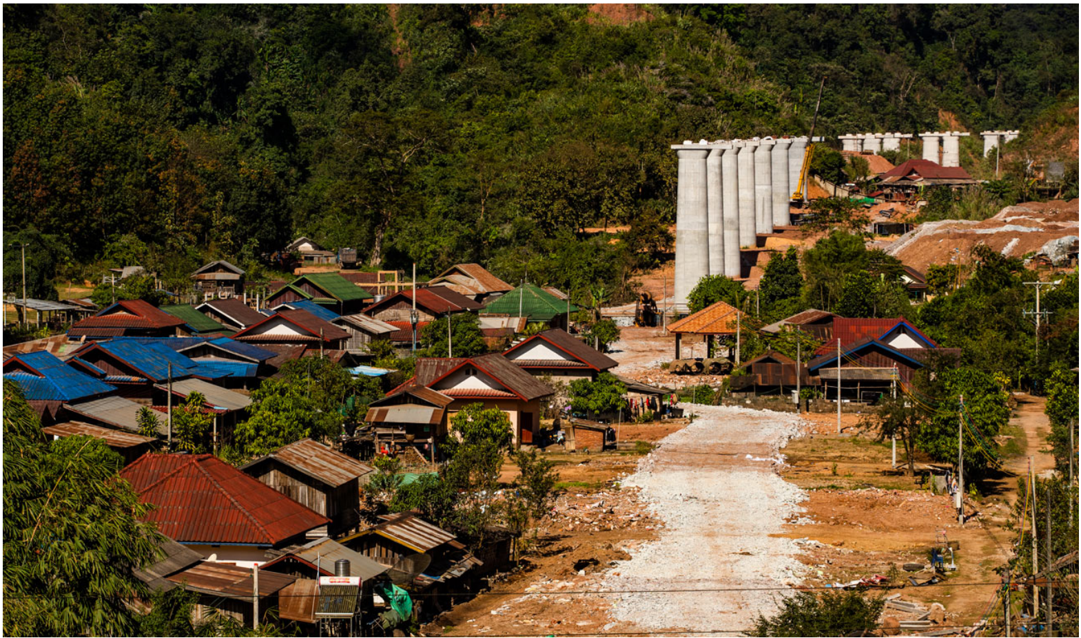
The construction of railway pylons for tracks to run above Bopiet or 'new village' (新家), 6 kilometres south of Boten SEZ. Photo by Carl Zoch, 2019.
